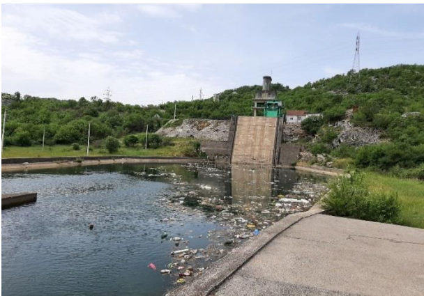
Picture 3. Drains - waste materials (especially plastic waste accumulates in parts of the reservoir and canals, and especially around the building.
