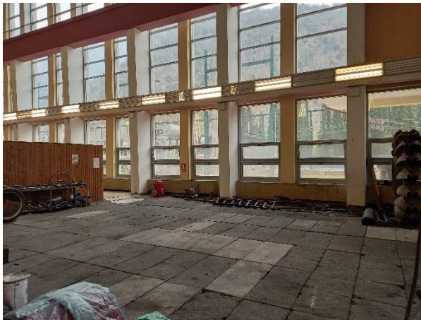
Place of instalacion of unit 8
